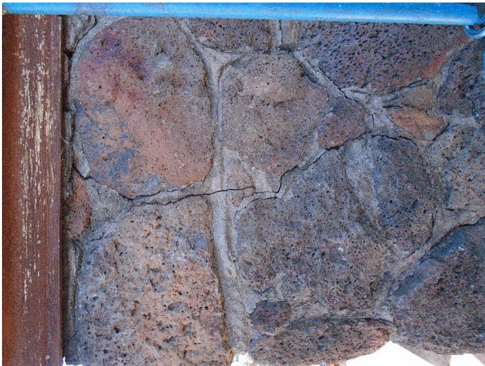
Photo 78 Isolated crack in volcanic rock.
