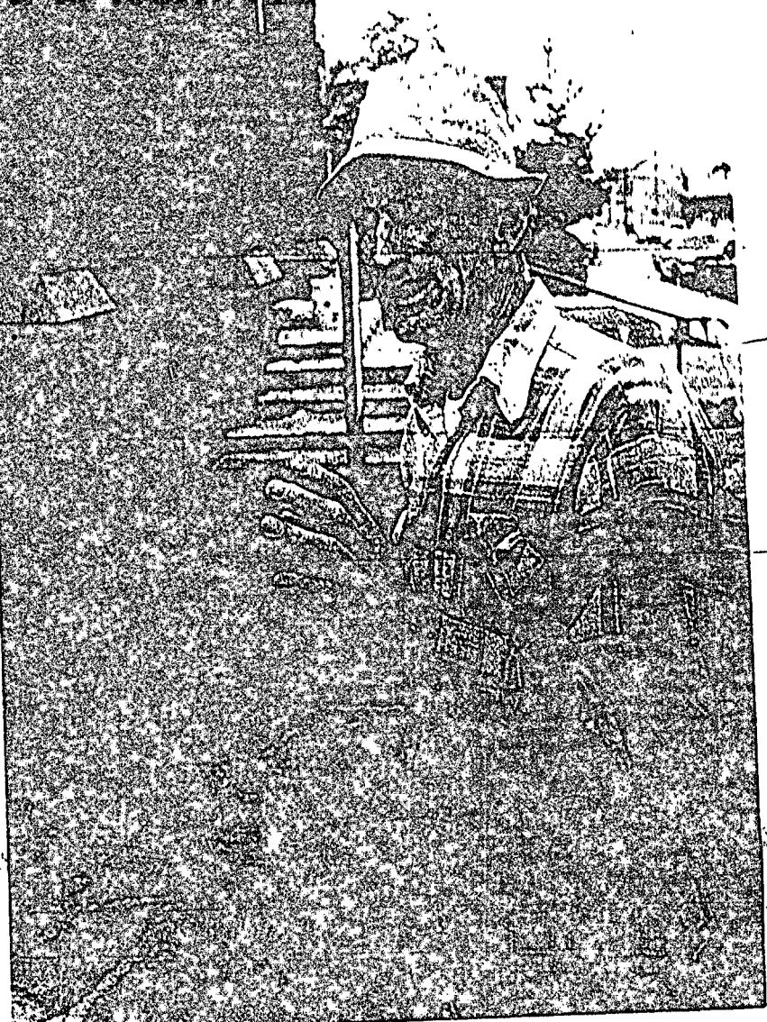
CHARLES SCOTT of Phoenix describes some of the techniques he is using to restore the Church of the Nativity of the Blessed Virgin Mary. Scott and two other men, John Dzielinski and Scott Bindon, have been working on the church for six weeks and work could continue for another 4-6 weeks. (SUNphoto)
